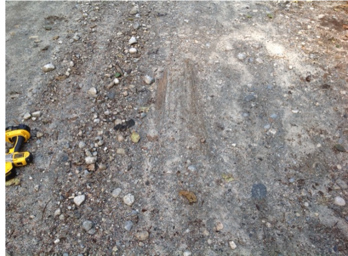
log stringer exposed
